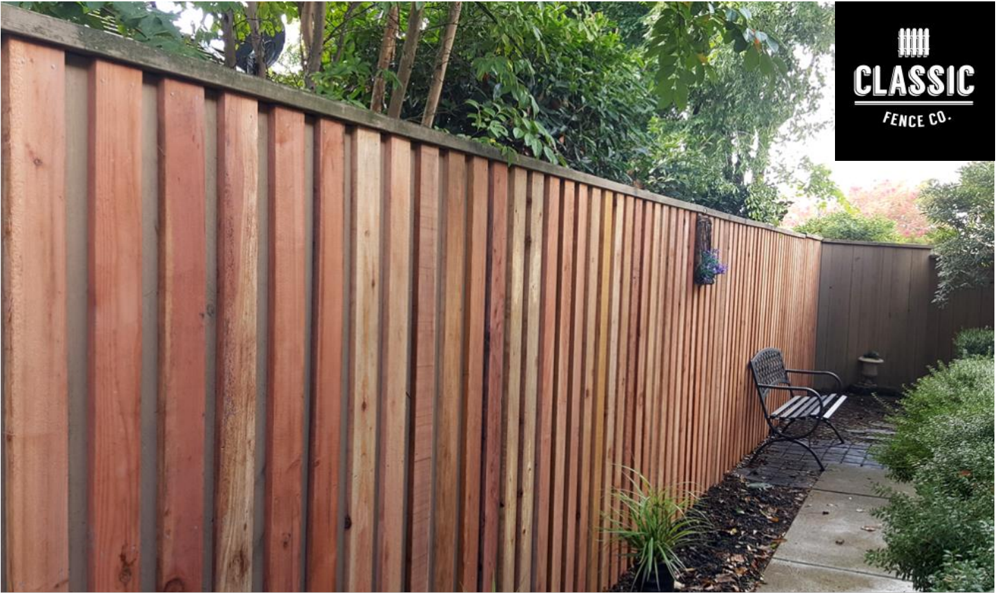
ADD 1X4 TO EXISTING FENCE TO COVER GAPS
